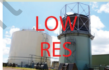
The large digester tanks used at the piggery for biogas production
