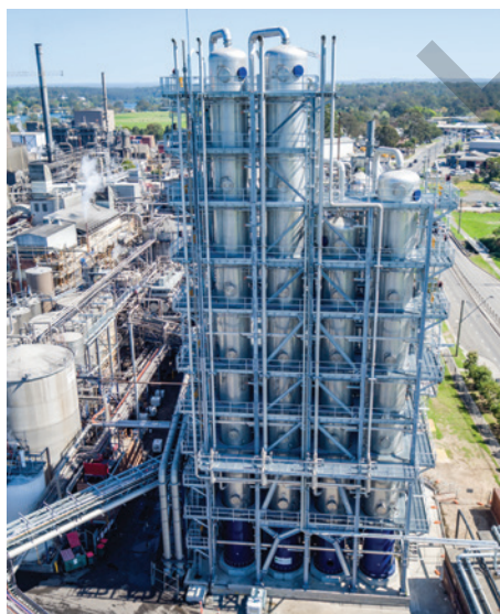
FIGURE 2.4.3 Tall distillation columns such as these ones at Manildra in NSW are common to all bioethanol plants.
