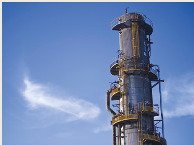
FIGURE 1.3.12 The distillation tower at an oil refinery
