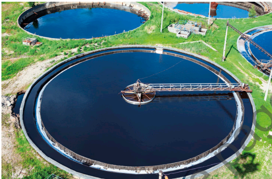
FIGURE 1.3.5 Sedimentation tanks are used in water treatment plants to separate solid waste from liquid waste.
